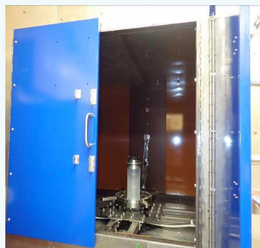
X-Ray Irradiation / Thermal Aging Facility
